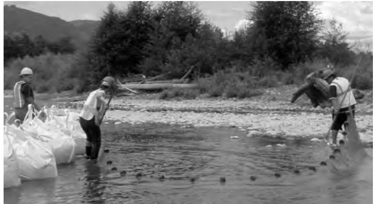
Russell Roberts, Treva Coe, and Francisco (Biscuits) Sanchez conducting fish exclusion before construction.
