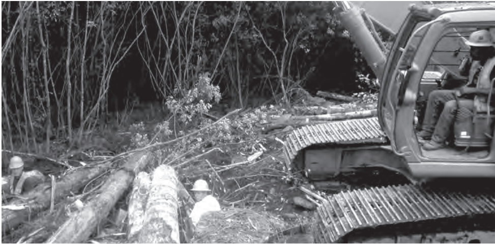
Darren Malloway, Sindick Bura, and Jeff Point clearing the way to install cable.
